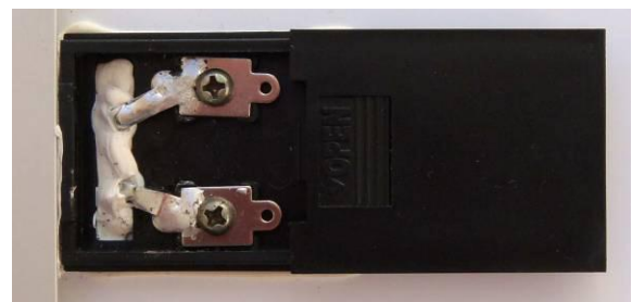
Open Junction Box
